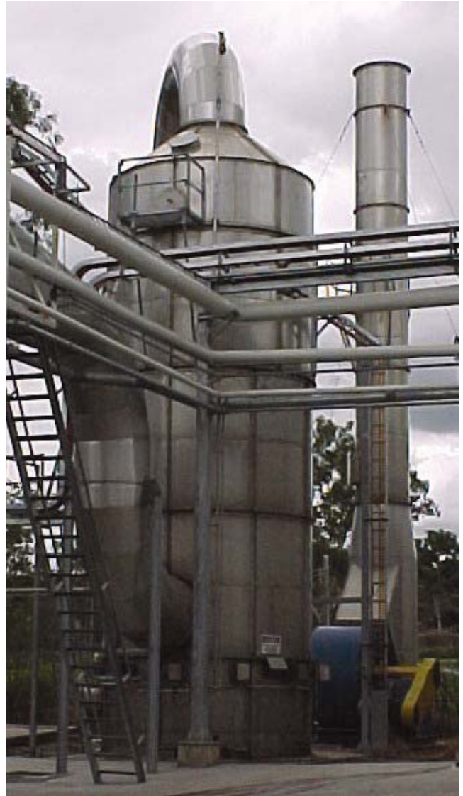
Figure 1. Packed tower scrubber.
