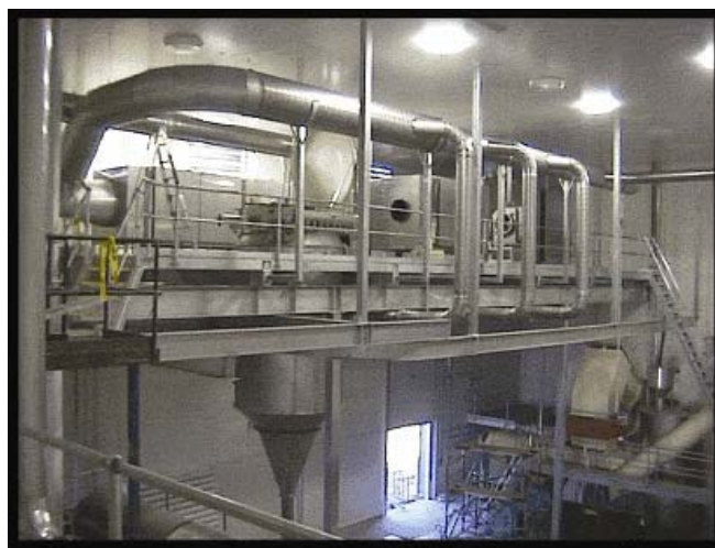
Figure 2. UV-C and Ozone treatment plant
